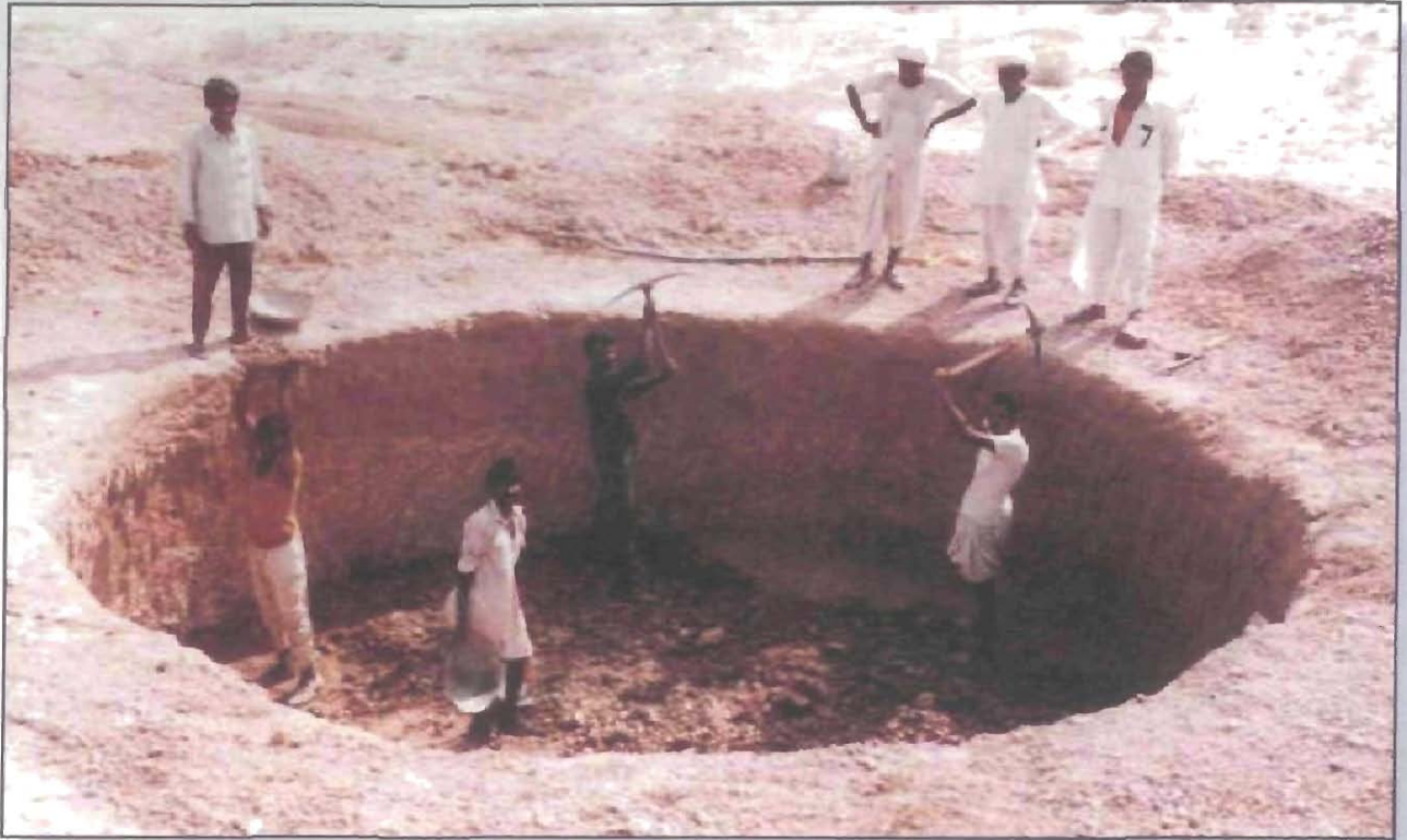
Construction of improved tanka (50,000 liters) with farmer's active participation at Kalyanpur (Distt. Barmer)
